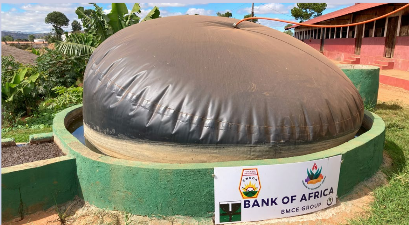
Main fermentation pit with its gas dome and the pipe transporting the produced gas to the school's kitchen
